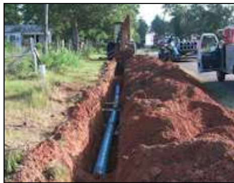
Photo 1: Water lines are under construction to replace the leaky distribution system that left the Cranberry community with insufficient water supply.
